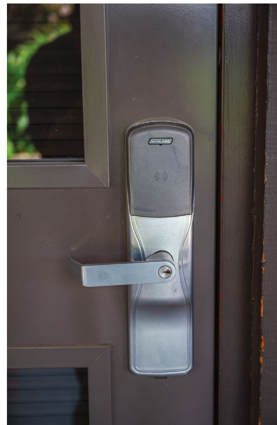
Allegion's Schlage Access Control at Irvine Valley College.
